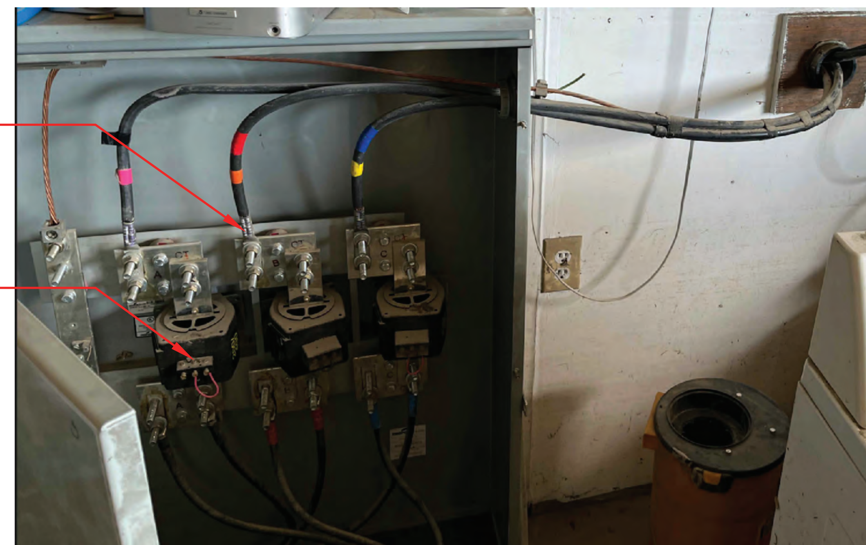
2 EXISTING FEEDER J-BOX TERMINATION PHOTO ER4 NO SCALE
