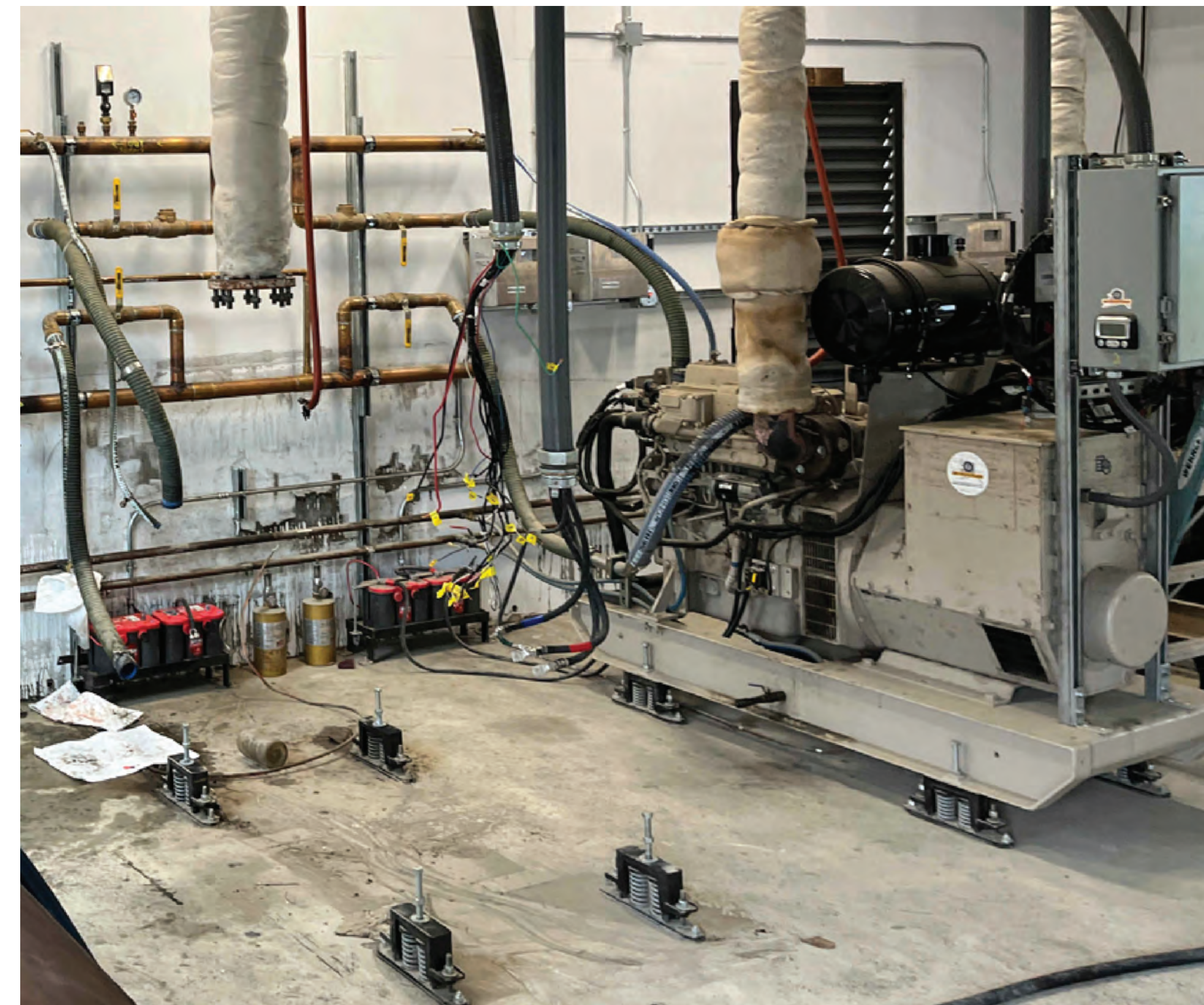
2 EXISTING GEN#1 (REMOVED) & GEN#2 (IN PLACE) REFERENCE PHOTO MR2 1"=1'-0"
