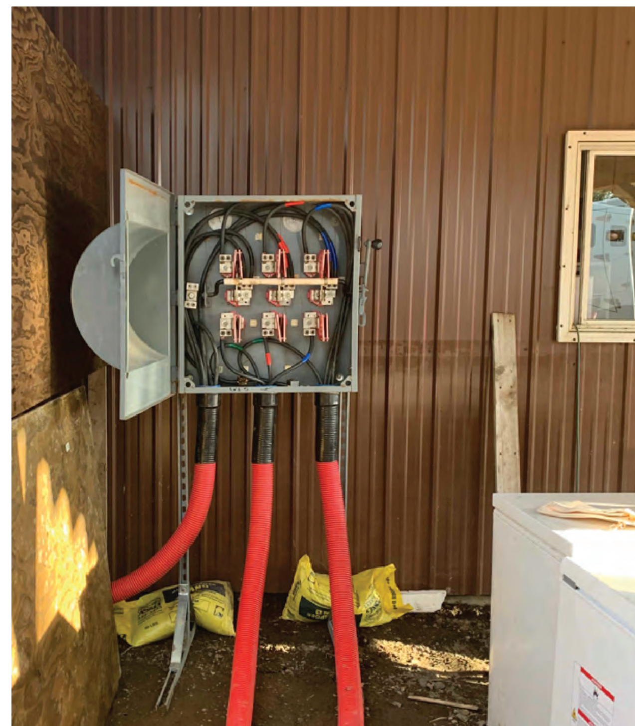
5 TRANSFER SWITCH LOCATION REFERENCE PHOTO ER3 3/4"=1'-0"
