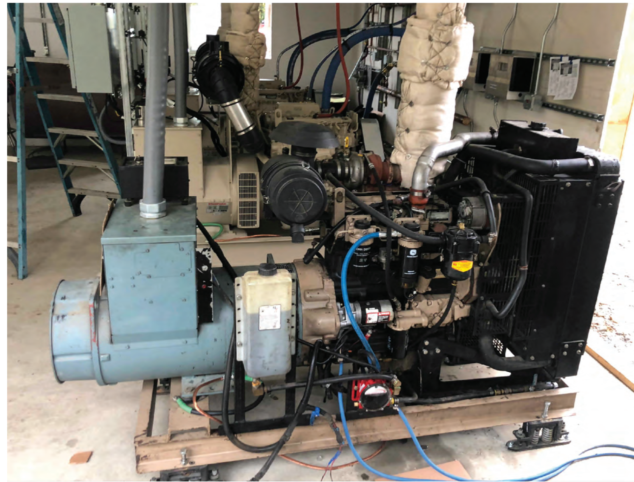
2 EXISTING GEN#3 REFERENCE PHOTO MR3 1"=1'-0"
