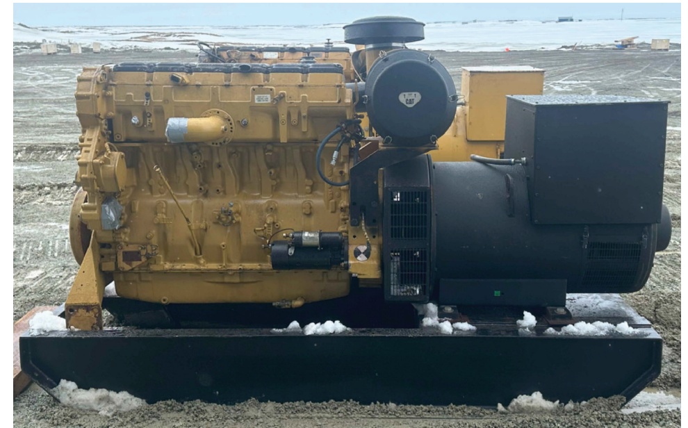
2 KIPNUK ENGINE-GENERATOR LEFT SIDE NO SCALE
