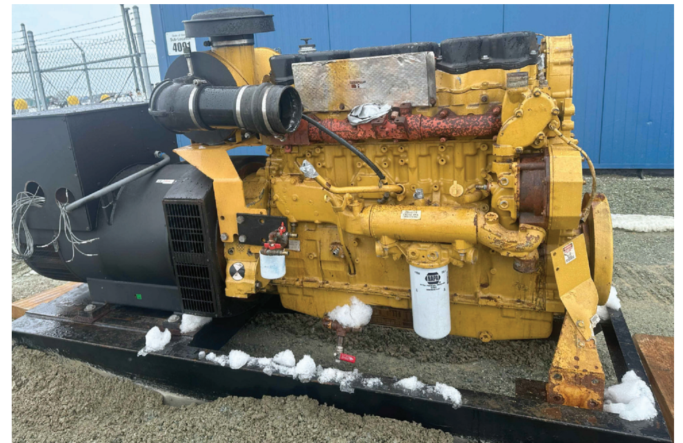
3 KIPNUK ENGINE-GENERATOR RIGHT SIDE NO SCALE
