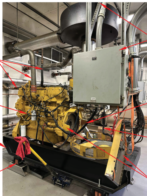
EXISTING GEN#2 LEFT SIDE PRIOR TO MODIFICATIONS
