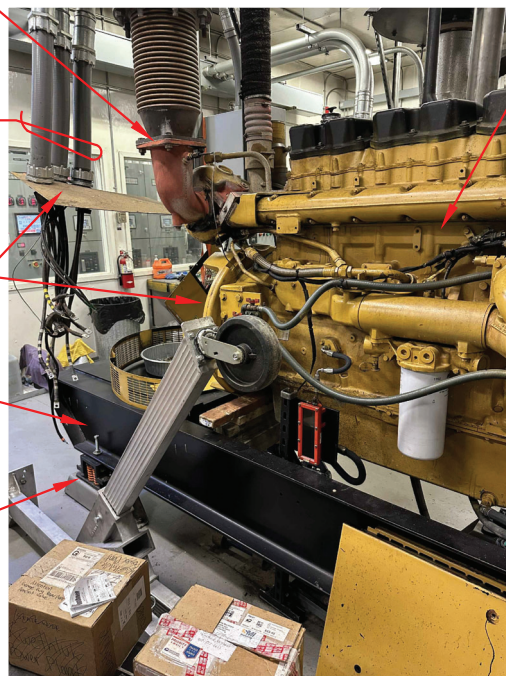
EXISTING GEN#2 RIGHT SIDE PRIOR TO MODIFICATIONS
