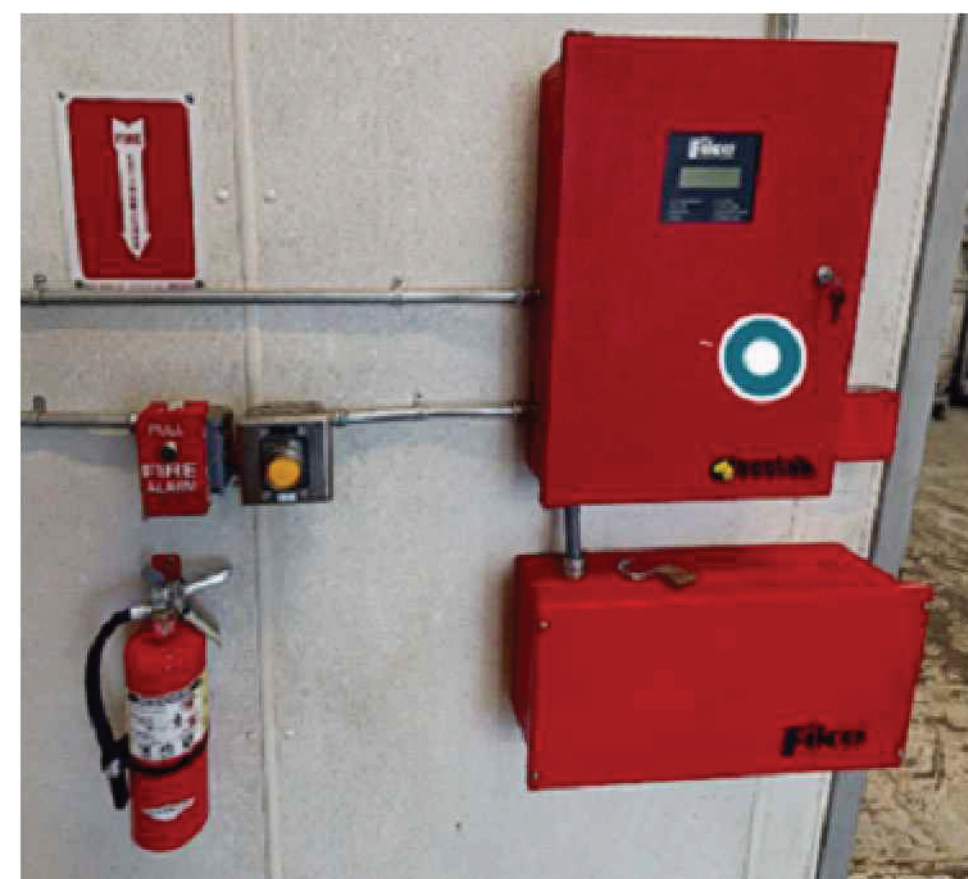
3 PHOTO OF PANEL & PULL STATION FS1 NO SCALE
