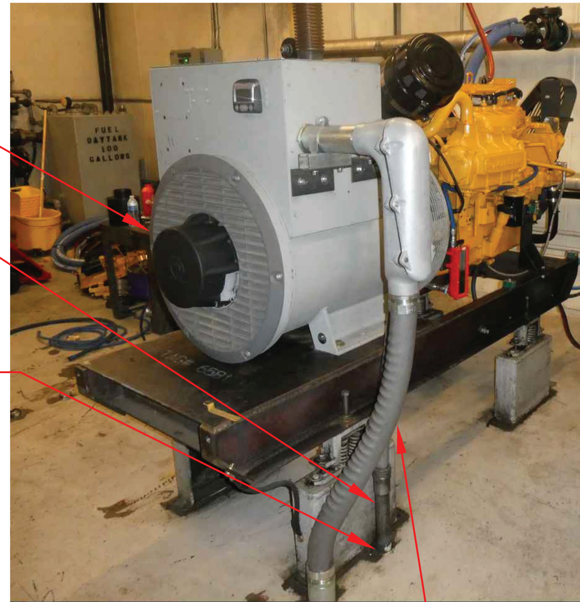
EXISTING GEN#3 PRIOR TO DEMOLITION
