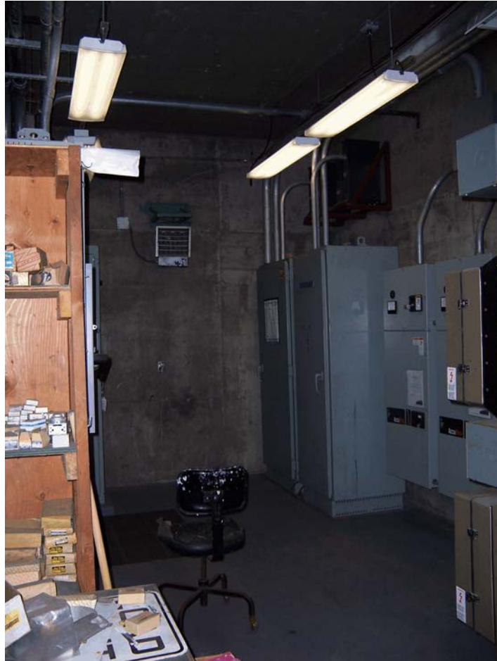
Interior of electrical room.
