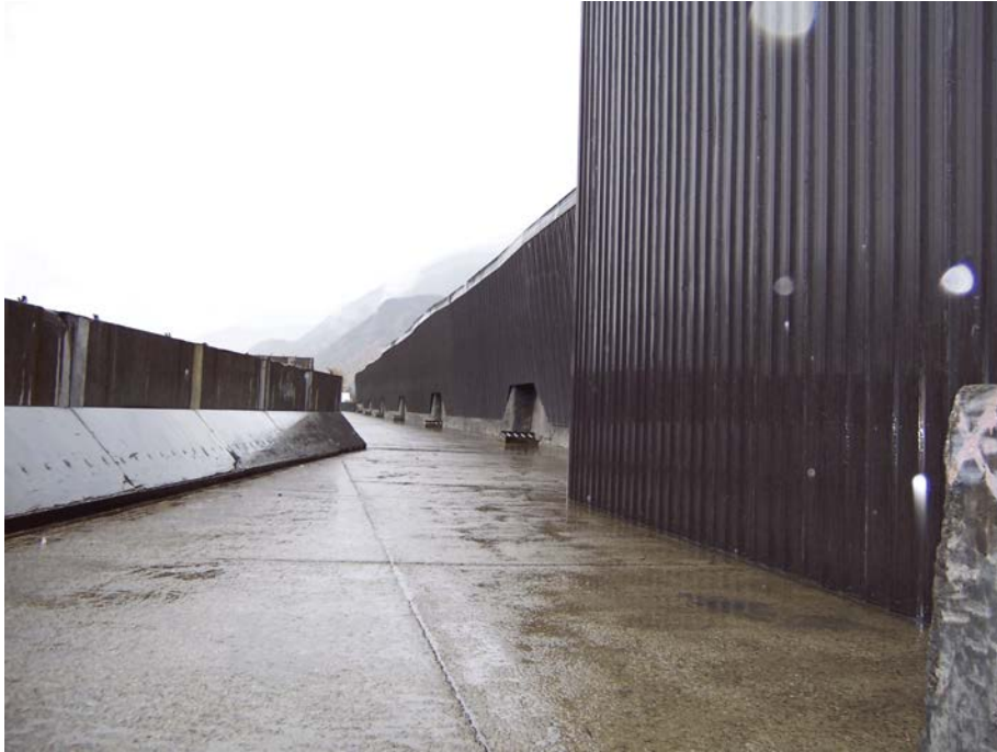
Looking along the reclaim conveyor building within the storage facility, looking in a northerly direction.
