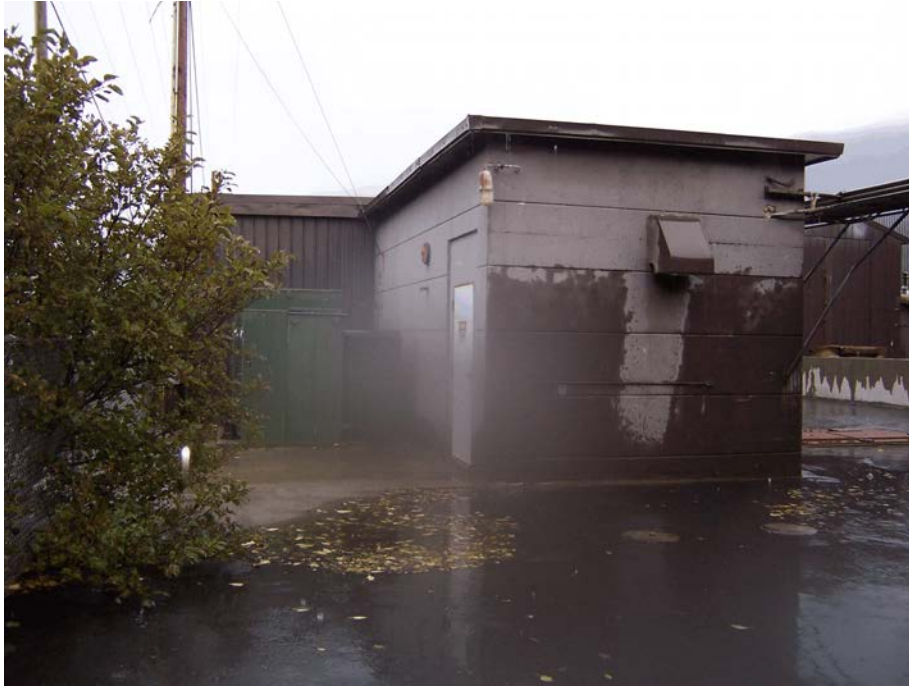
Electric transformer building referred to on map as MCC.
