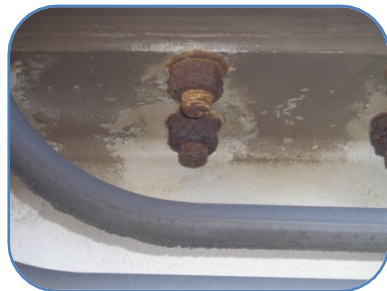
Extremely Corroded Bolts
