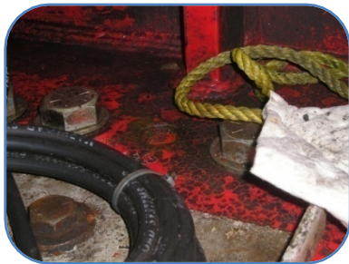
Missing Slew (Swing) Bolt
