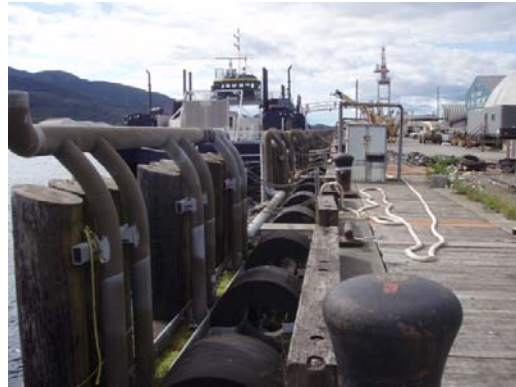
Top of Fender Main Berth
