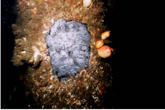
Cleaned Pile Galvanizing Gone
