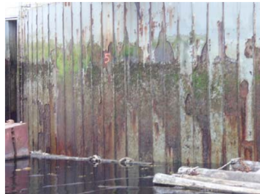
Cell 5 Note coating failure
