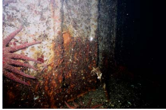
Typical cell at mudline. Note coating gap
