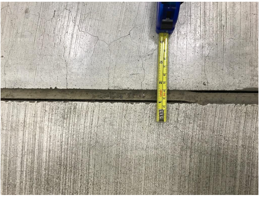
Photo 3 - Crack between sealant and joint
