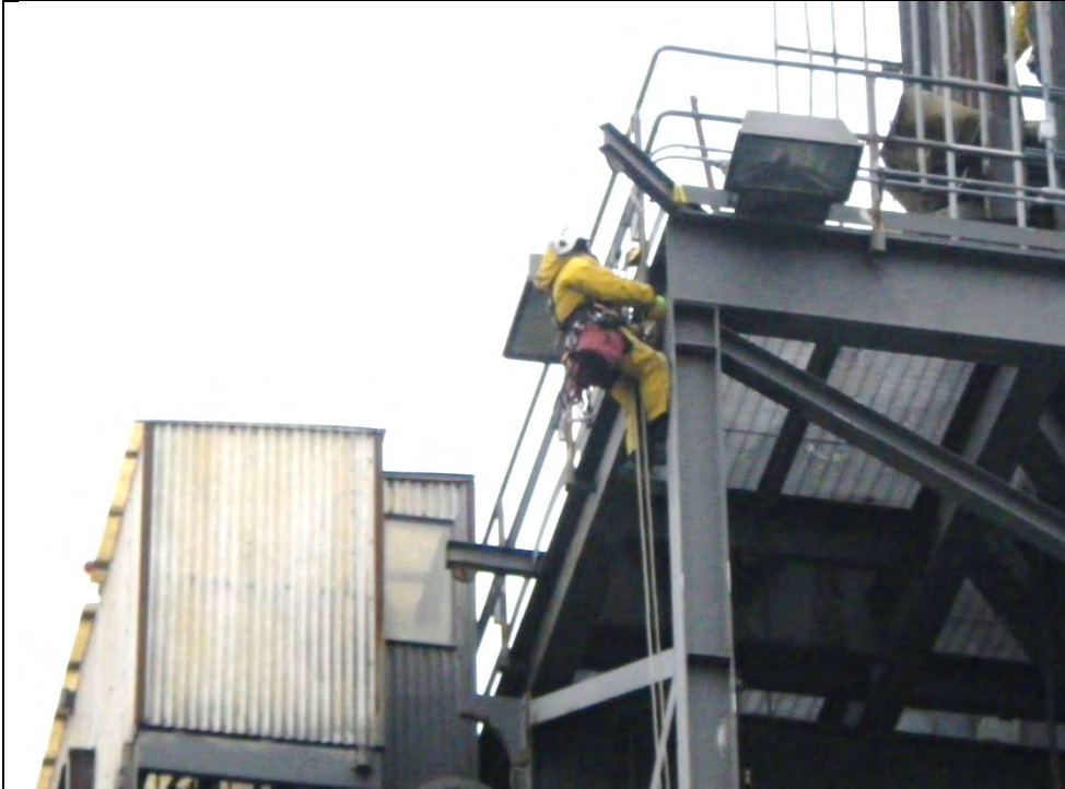
JKM-111213-IMG0287 LOCATION: SKAGWAY ORE TERMINAL SHIP LOADER DESCRIPTION: CLOSEUP VIEW OF INSPECTOR AT TOP OF SW COLUMN OF SOUTH TOWER. HYDRAULIC EQUIPMENT HOUSE AT LEFT.
