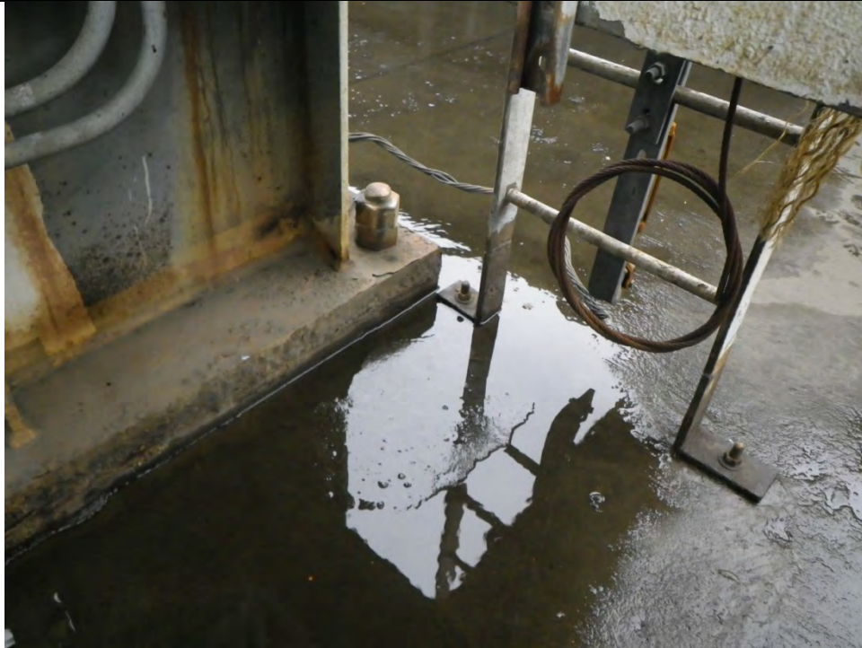
JKM-111213-IMG0411 LOCATION: SKAGWAY ORE TERMINAL SHIP LOADER DESCRIPTION: BASE OF SW COLUMN OF NORTH TOWER OF SHIP LOADER
