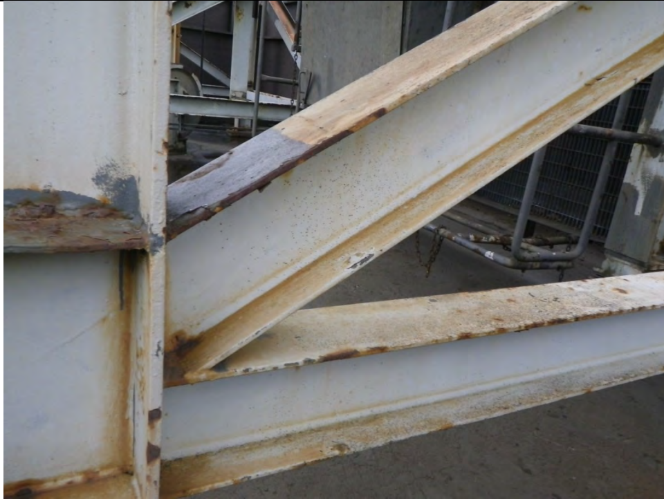
JKM-111213-IMG0372 LOCATION: SKAGWAY ORE TERMINAL SKAGWAY ORE TERMINAL DESCRIPTION: SOUTH TOWER NW COLUMN FRAMING IN NORTH FACE OF TOWER
