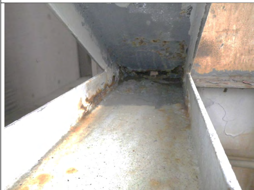
JKM-111213-IMG0403 LOCATION: SKAGWAY ORE TERMINAL SHIP LOADER DESCRIPTION: TOWER FRAME CONNECTION, NOTE DRAIN HOLE
