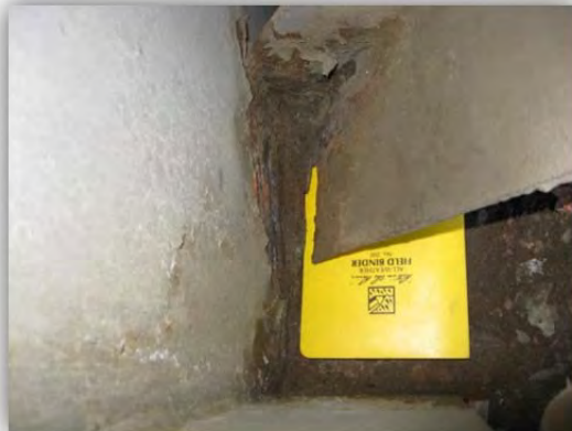
Example of extreme CS5 deteriorated condition in boom conveyor support framing
