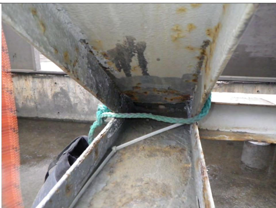
JKM-111213-IMG0409 LOCATION: SKAGWAY ORE TERMINAL SHIP LOADER DESCRIPTION: FRAME CONNECTION AT BASE OF WEST FACE OF NORTH TOWER OF SHIP LOADER; NOTE DRAIN HOLE IN "POCKET" FORMED BY WF FLANGES
