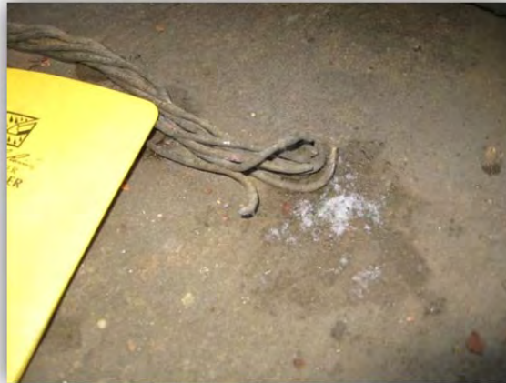
Example of partially failed ground strap at column base; CS5
