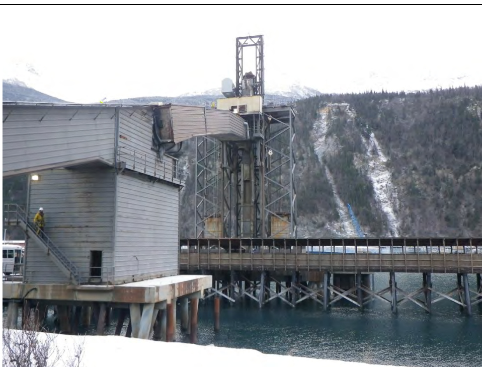
JKM-111313-IMGP0439 LOCATION: SKAGWAY ORE TERMINAL SHIP LOADER DESCRIPTION: SHIP LOADER AND TRANSFER CONVEYOR VIEWED FROM SHORE TO WEST OF THE ORE DOCK; INSPECTOR DESCENDING STAIWAY FROM DRIVE DECK TO BASE OF SUPPORT TOWER.
