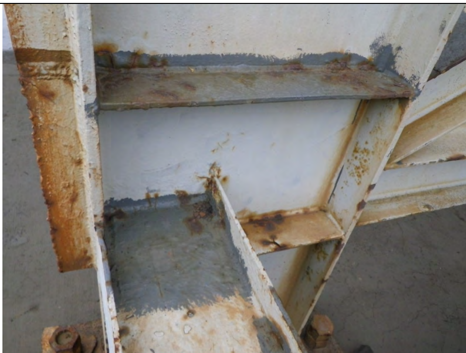
JKM-111213-IMG0371 LOCATION: SKAGWAY ORE TERMINAL SHIP LOADER DESCRIPTION: SOUTH TOWER NW COLUMN AND FRAMING CONNECTION
