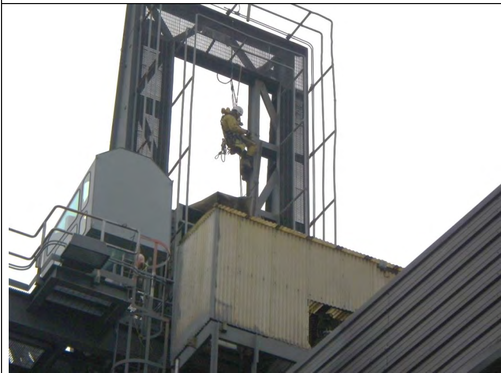
JKM-111213-IMG0283 LOCATION: SKAGWAY ORE TERMINAL SHIP LOADER DESCRIPTION: INSPECTOR RIGGED OFF OF SHIP LOADER BOOM CROSS FRAME BEGINNING BOOM STRUCTURAL INSPECTION.
