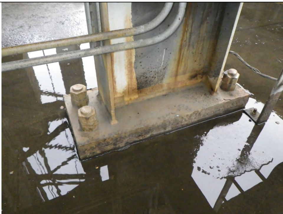
JKM-111213-IMG0410 LOCATION: SKAGWAY ORE TERMINAL SHIP LOADER DESCRIPTION: BASE OF SW COLUMN OF NORTH TOWER OF SHIP LOADER
