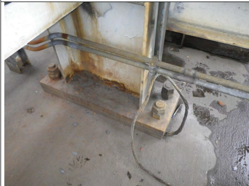
JKM-111213-IMG0404 LOCATION: SKAGWAY ORE TERMINAL SHIP LOADER DESCRIPTION: BASE OF SE COLUMN NORTH TOWER
