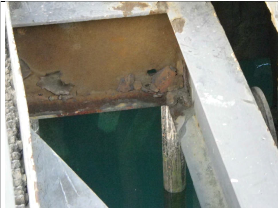
JKM-111313-IMGP0471 LOCATION: SKAGWAY ORE TERMINAL SHIP LOADER BOOM DESCRIPTION: LATERAL SUPPORT FROM RIGHT (SOUTH) BOOM GIRDER TO RIGHT SHUTTLE SUPPORT BEAM/RUNWAY
