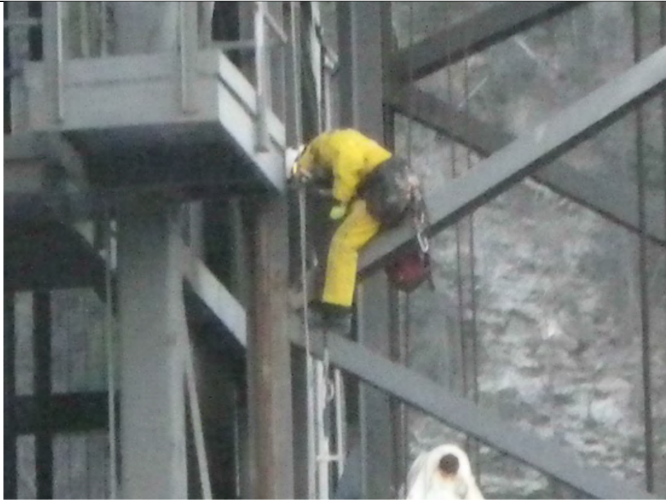
JKM-111313-IMG0442 LOCATION: SKAGWAY ORE TERMINAL SHIP LOADER DESCRIPTION: INSPECTOR ON SE COLUMN OF NORTH TOWER
