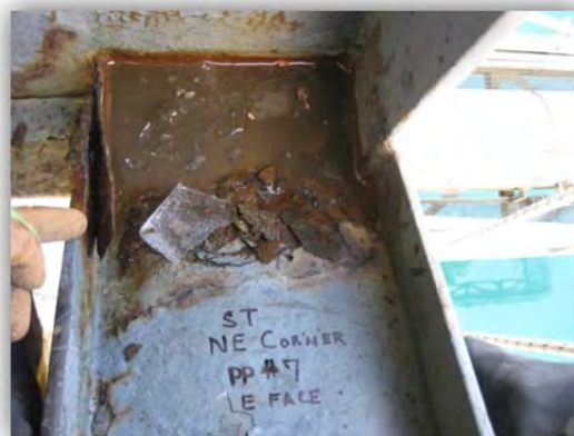
Typical tower frame joint of configuration that pools water; CS5.
