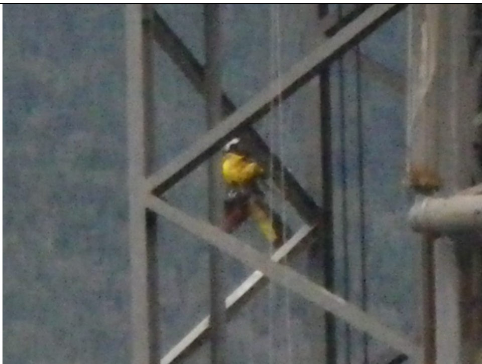
JKM-111213-IMG0428 LOCATION: SKAGWAY ORE TERMINAL SHIP LOADER DESCRIPTION: INSPECTOR ON SOUTH FACE OF SOUTH TOWER, INSPECTING STEEL MEMBERS AND CONNECTIONS
