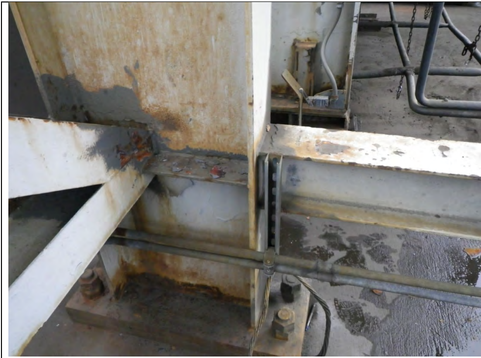
JKM-111213-IMG0405 LOCATION: SKAGWAY ORE TERMINAL SHIP LOADER DESCRIPTION: NORTH TOWER BASE SE COLUMN, FRAMING AND BASE PLATE
