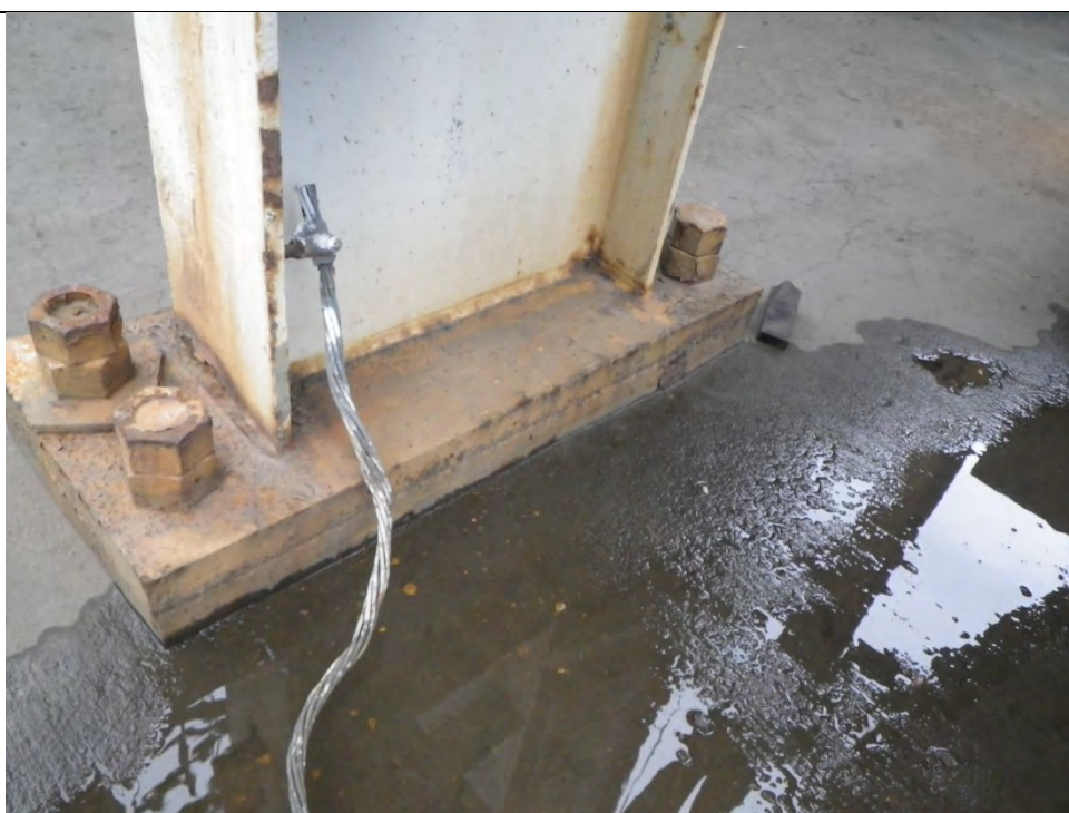
JKM-111213-IMG0370 LOCATION: SKAGWAY ORE TERMINAL SHIP LOADER DESCRIPTION: SOUTH TOWER NW COLUMN BASE SOUTH FACE
