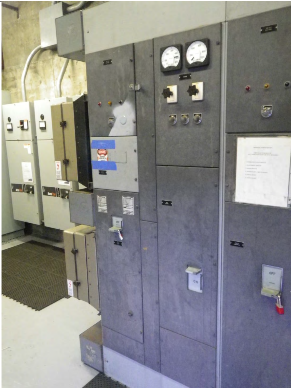
JKM-111313-IMG0441 LOCATION: SKAGWAY ORE TERMINAL SHIP LOADER DESCRIPTION: SHIP LOADER POWER DISCONNECT IN MAIN MCC (MCC NO. 1) LOCKED OUT/TAGGED OUT
