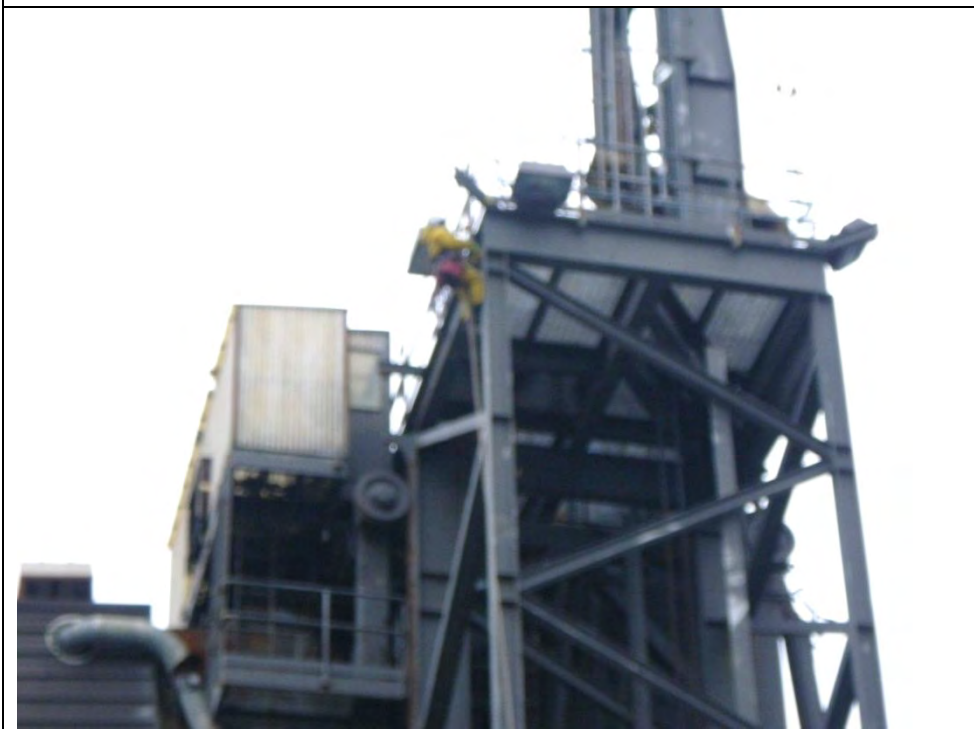
JKM-111213-IMG0286 LOCATION: SKAGWAY ORE TERMINAL SHIP LOADER DESCRIPTION: INSPECTOR AT TOP OF SW COLUMN OF SOUTH TOWER. HYDRAULIC EQUIPMENT HOUSE AT LEFT.
