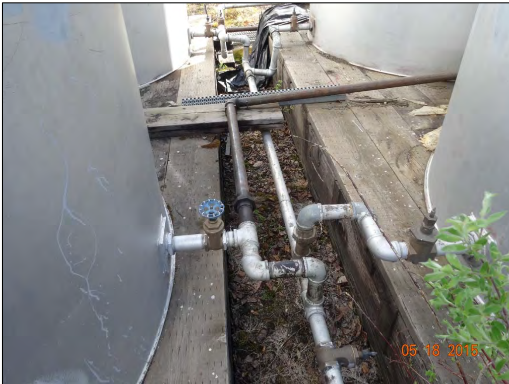
Photo 2 – School Tanks Manifold Piping
