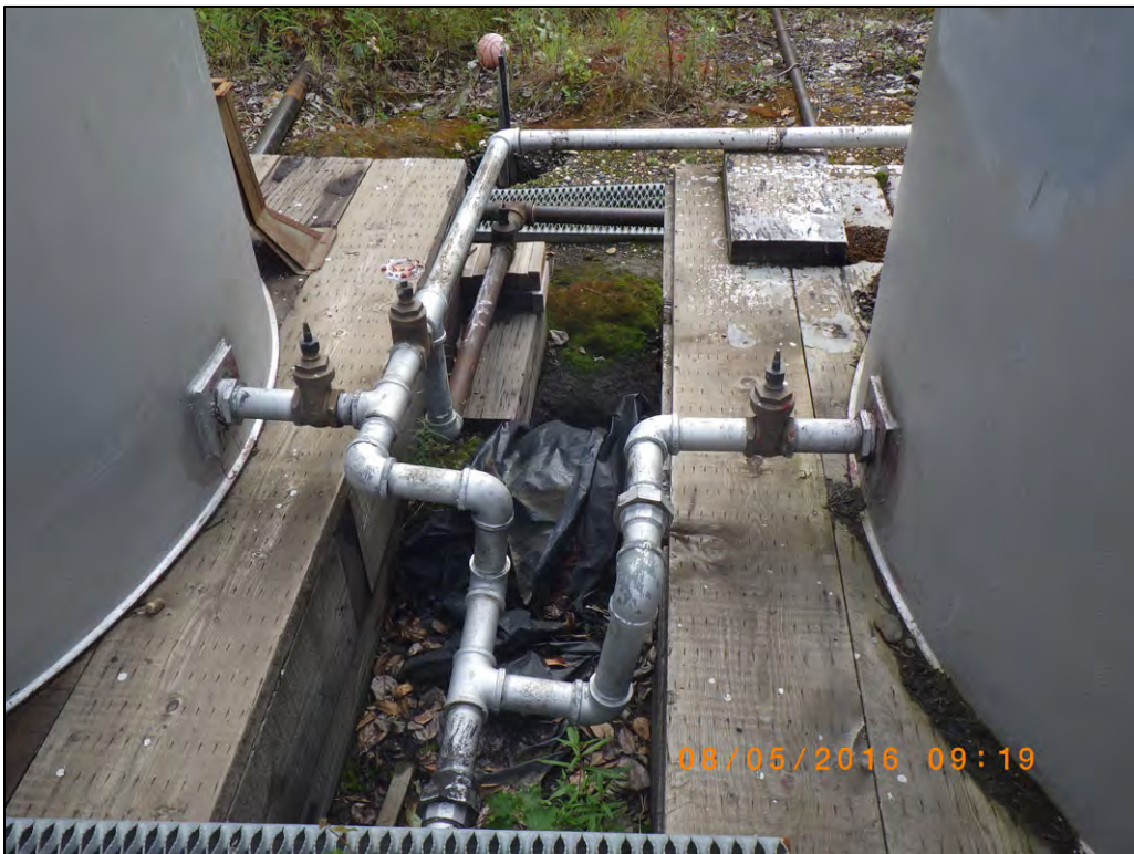
Photograph 5: Tank Farm #1 manifold piping
