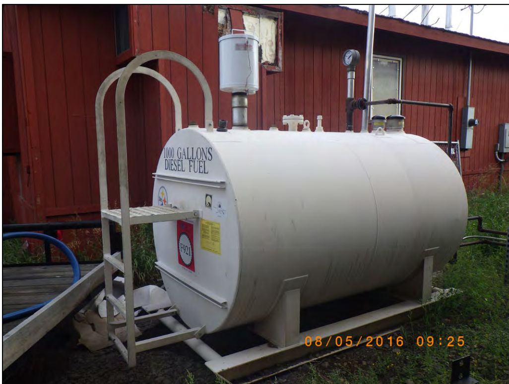
Photograph 14: generator house supply tank
