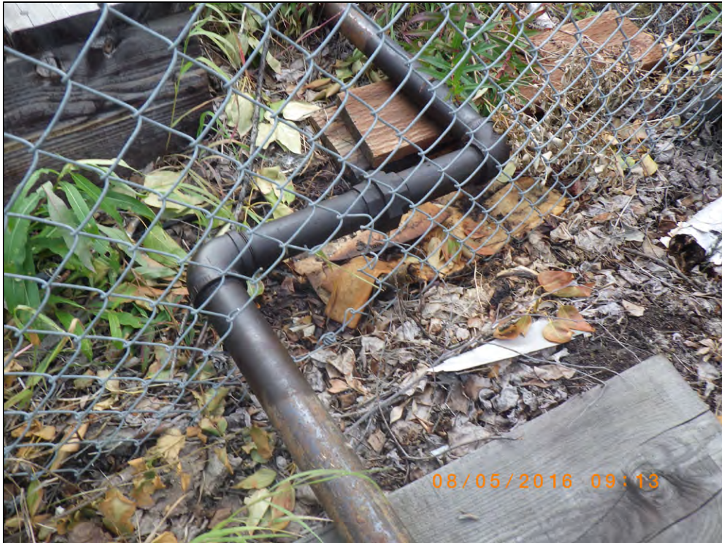
Photograph 6: Leaking feed pipe from Tank Farm #1 to the maintenance shop; no containment
