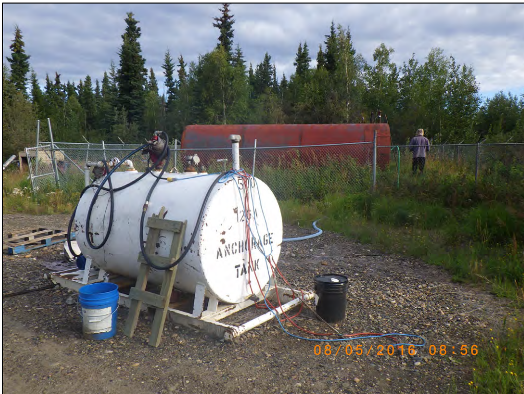
Photograph 12: 500 gal intermediate tank used to transfer fuel into the fuel trailer tank
