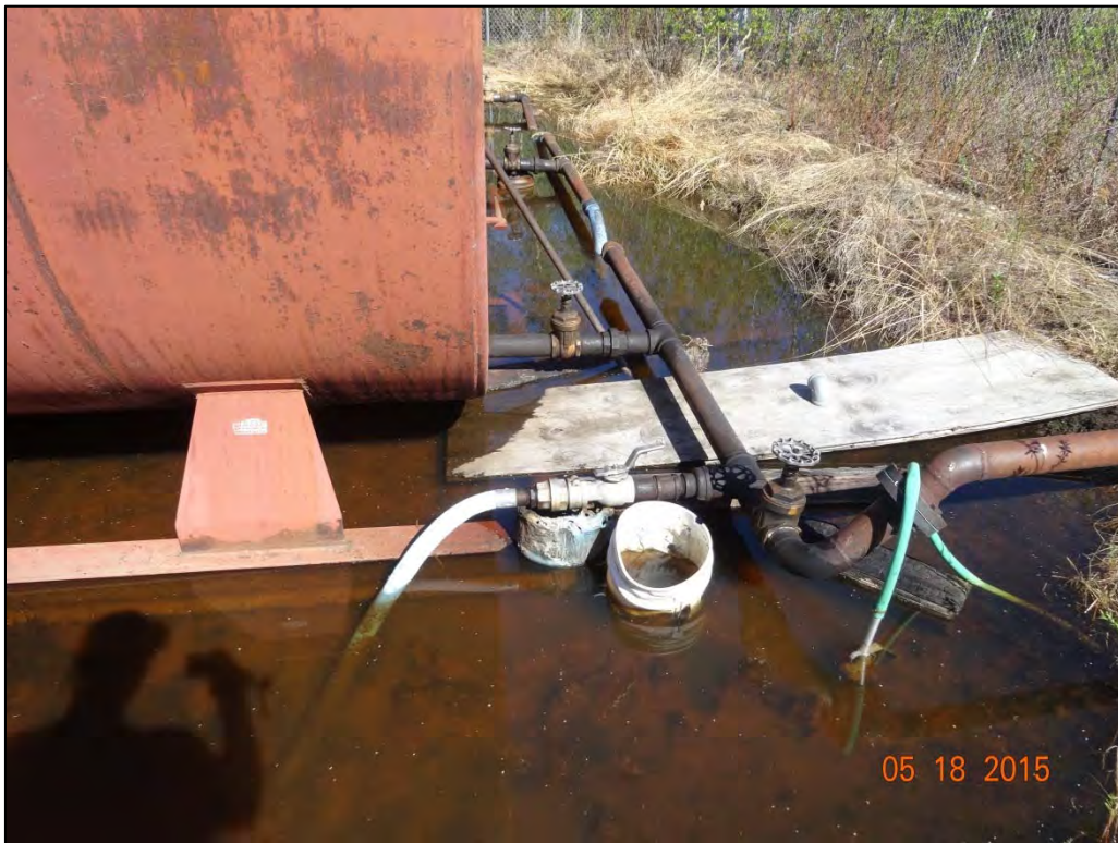
Photo 2 – Tank Farm 2 Piping and Inundated containment
