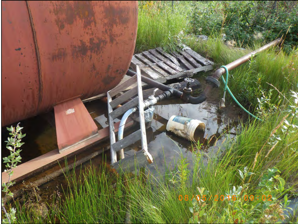
Photograph 11: Tank Farm #2 manifold piping
