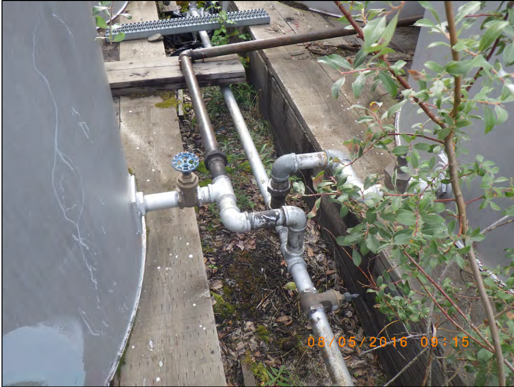
Photograph 4: Tank Farm #1 manifold piping
