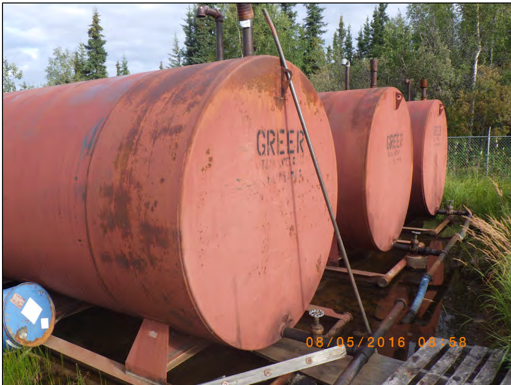
Photograph 10: Tank Farm #2 Beaver Village tanks; only tank #1 in foreground is in service
