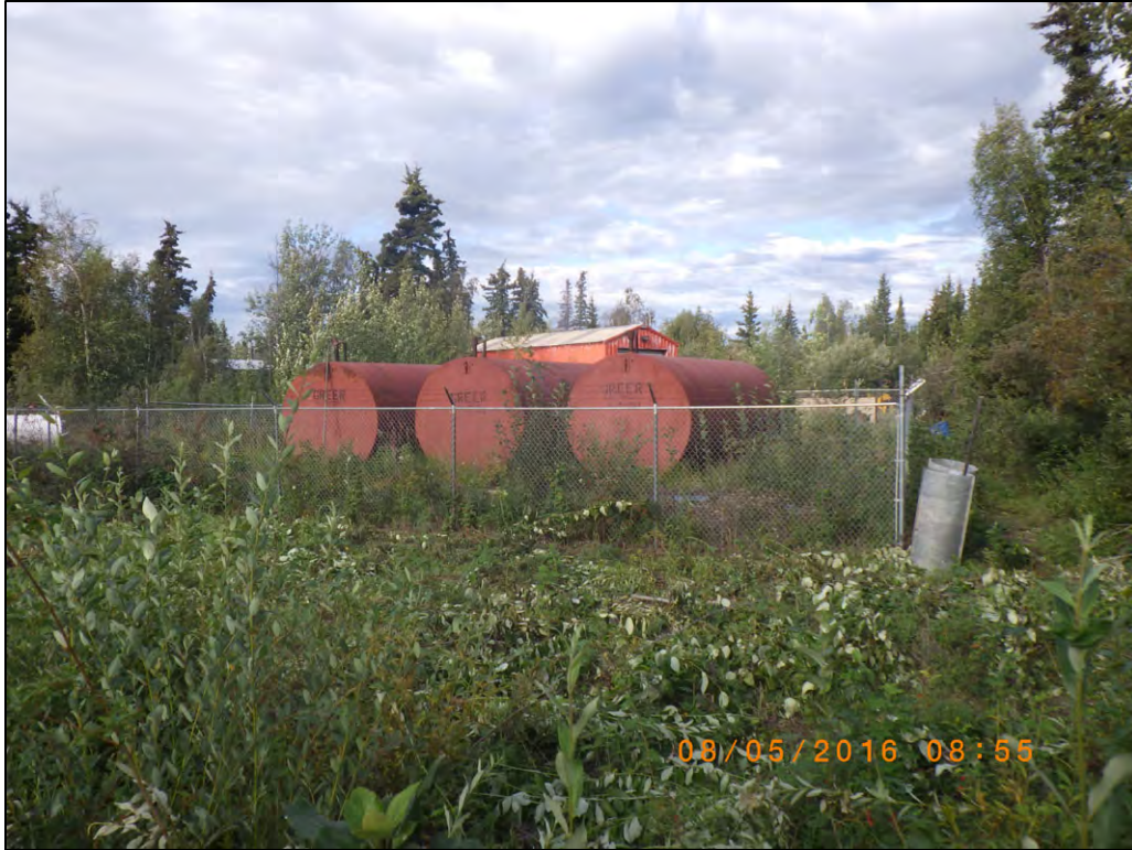
Photograph 9: Tank Farm #2 Beaver Village tanks
