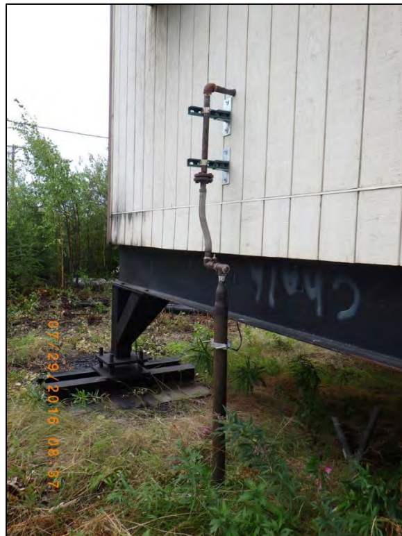
Photograph 8: Tank Farm #1 power plant feed line
