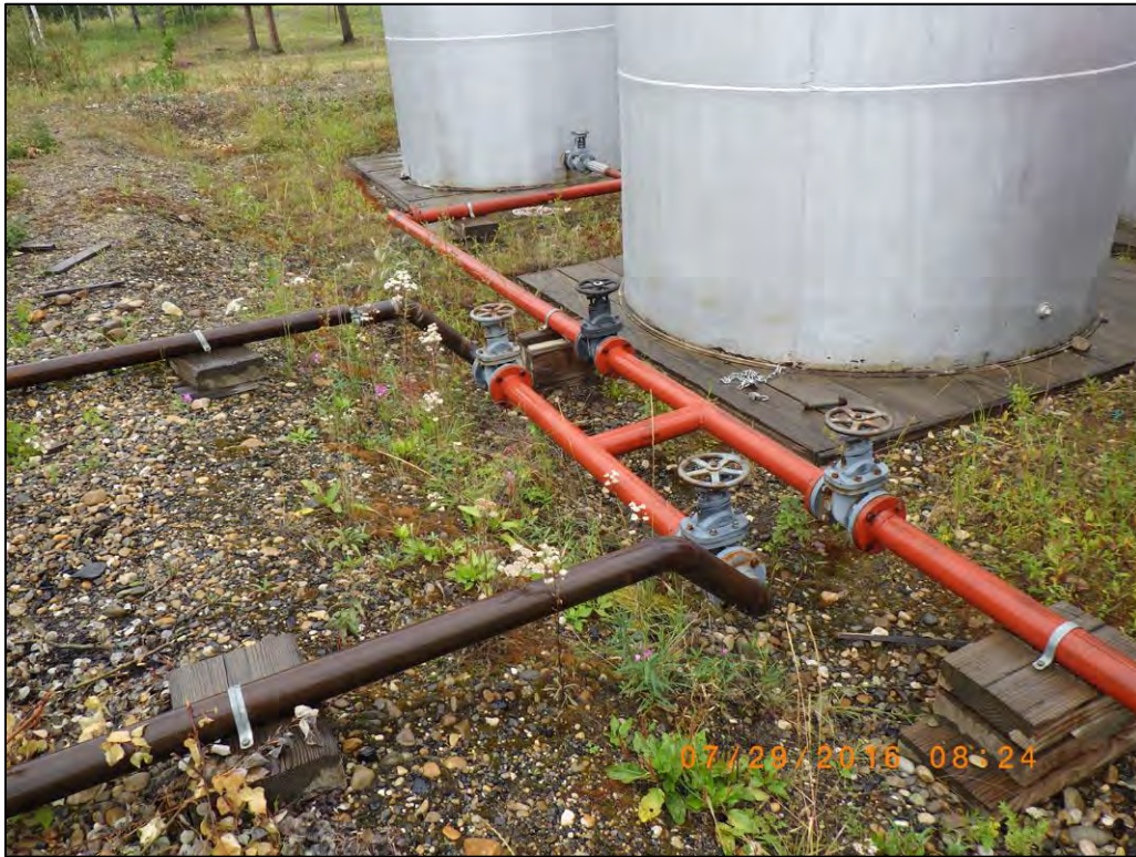
Photograph 3: Tank Farm #1 fill line manifold
