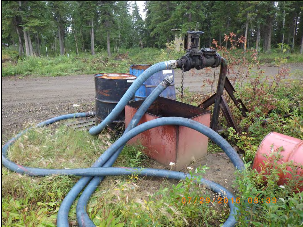
Photograph 1: Tank Farm #1 Airstrip Fill Header
