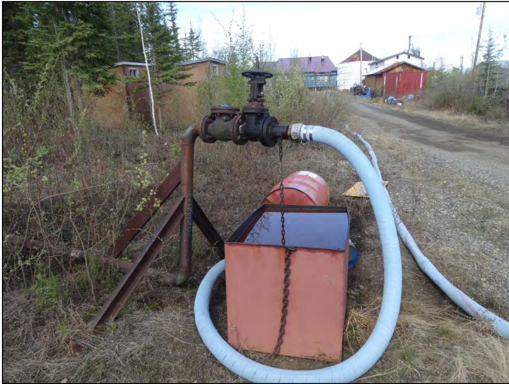
Photo 1 – Tank Farm 1 Airport Header
