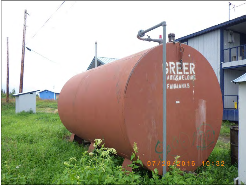
Photograph 11: Tank Farm #2 dispenser feed piping
