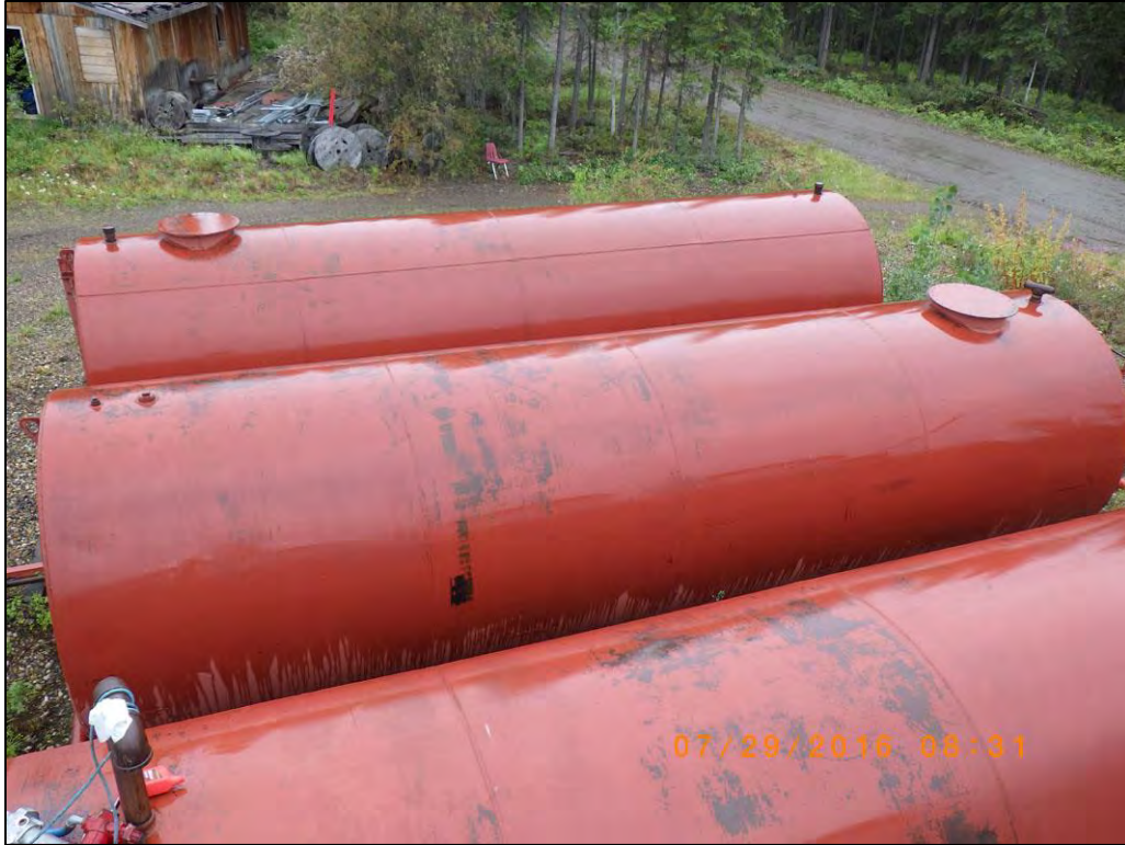
Photograph 7: Tank Farm #1 power plant tanks
