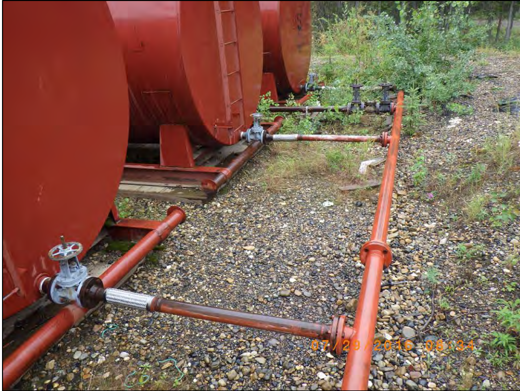
Photograph 5: Tank Farm #1 power plant tanks manifold
