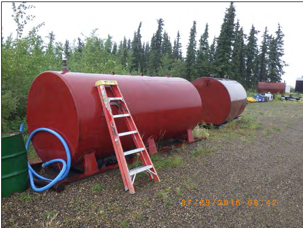
Photograph 14: Tank Farm #4 airstrip tanks; tank in background not-in-service
