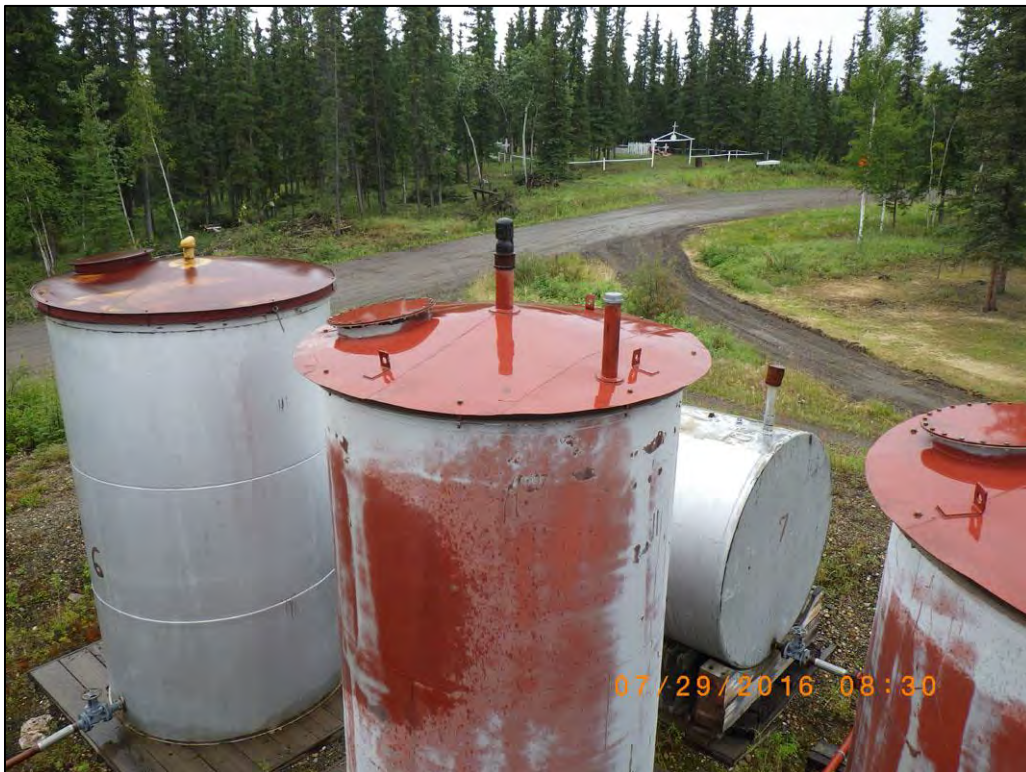
Photograph 6: Tank Farm #1 school tanks
