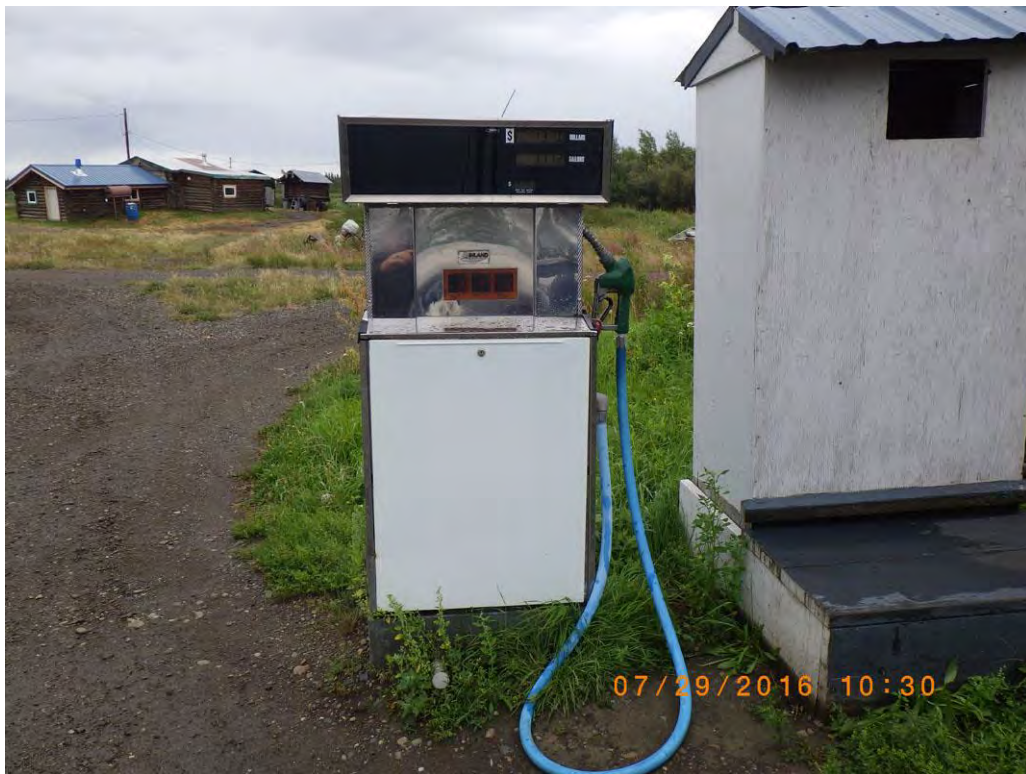
Photograph 12: Tank Farm #2 dispenser
