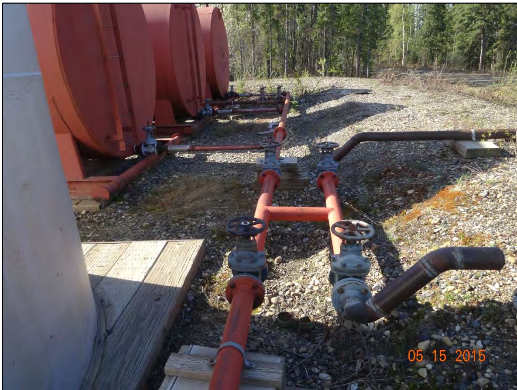
Photo 4 – Manifold for Power Plant Tanks
