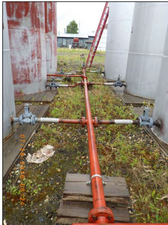
Photograph 4: Tank Farm #1 school tanks manifold
