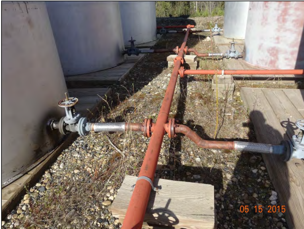
Photo 3 – Manifold For School Tanks
