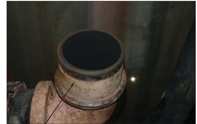
PROVIDE 4" FLANGED X 18" LONG ENGINE EXHAUST FLEX WITH COUPLING TO MATCH EXISTING EXHAUST CONNECTION 5 EXISTING E-GEN EXHAUST CONNECTION FITTING M2.3 NO SCALE
