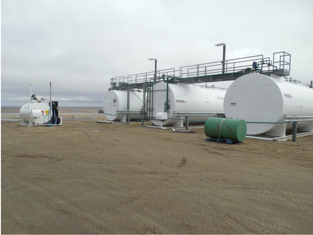
Photo 1 – Scammon Bay School Bulk Fuel Tanks
