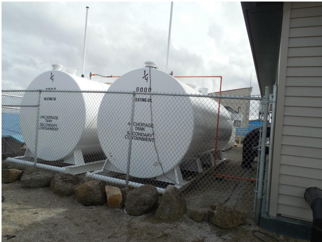
Photo 2 –City WTP Tank Farm
