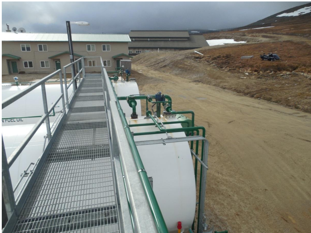
Photo 2 – Top of Tanks
