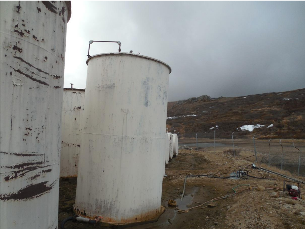
Photo 2 – Leaning Tank and Dike Settlement
