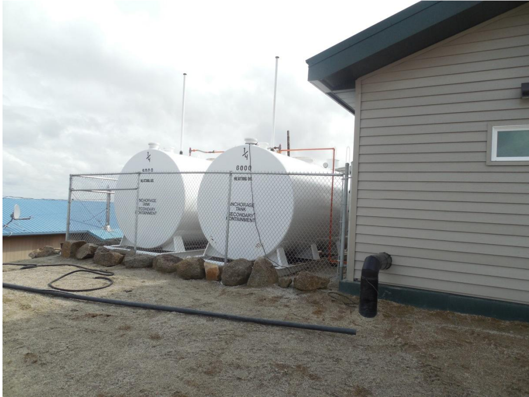
Photo 1 –City WTP Tank Farm
