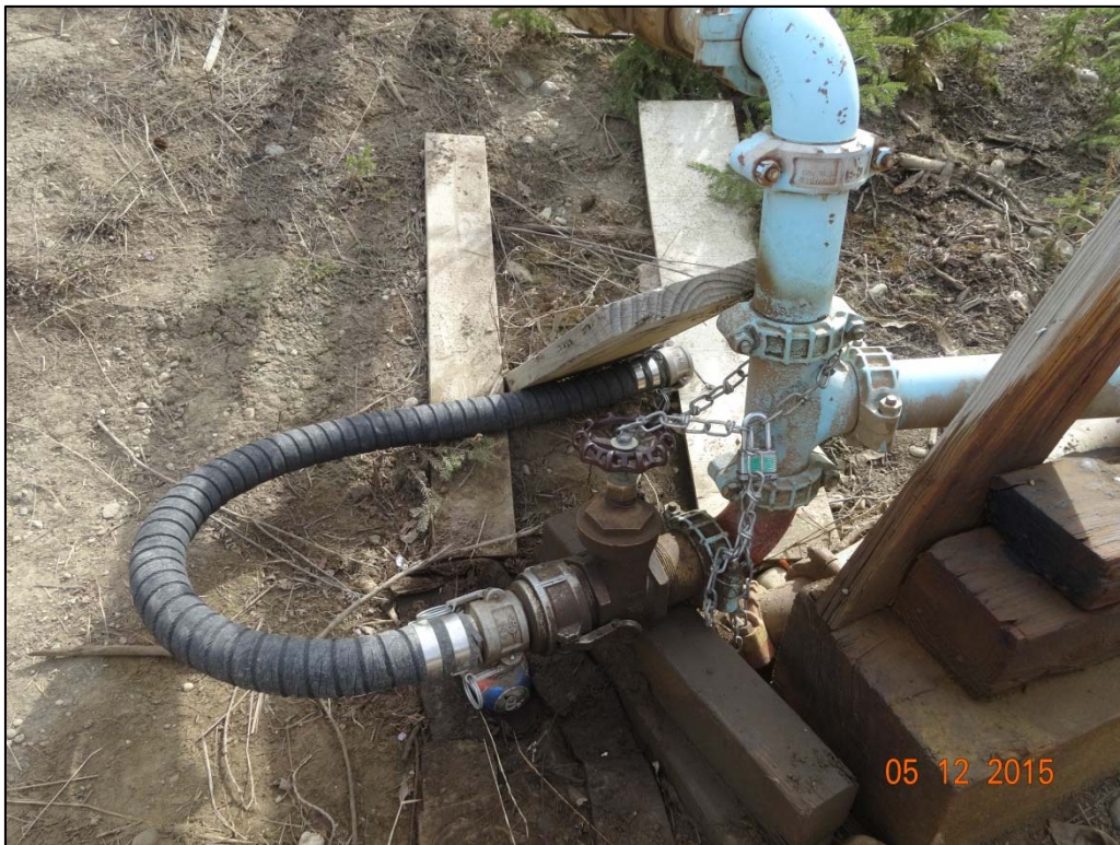
Photo 2 – Venetie School Tank Farm Truck Fill Header
