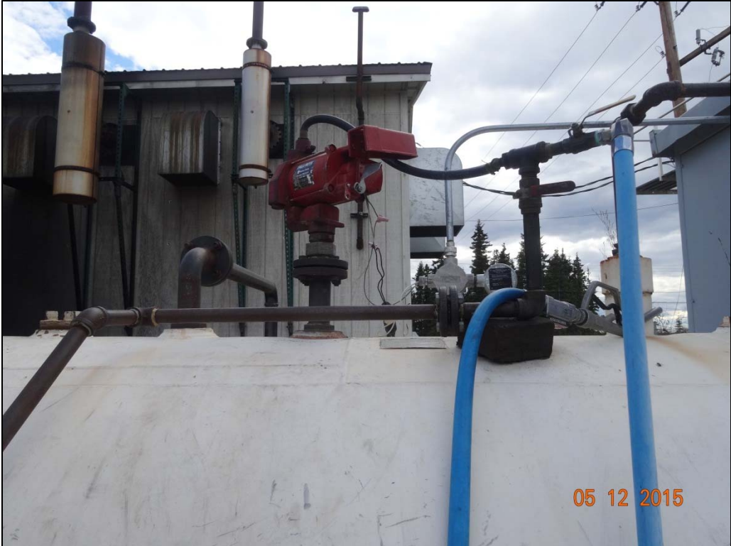
Photo 2 – Jury-Rigged Dispensing Pump on Tank 3
