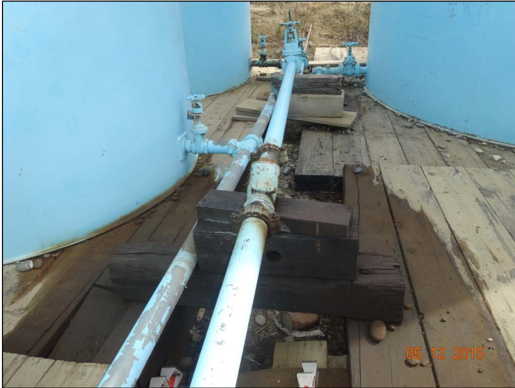
Photo 3 – Weeping Victaulic Fittings in Manifold
