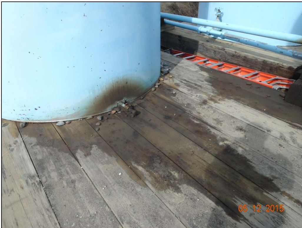
Photo 4 – Fuel Staining Emanating from Threaded Water Drain Fitting
