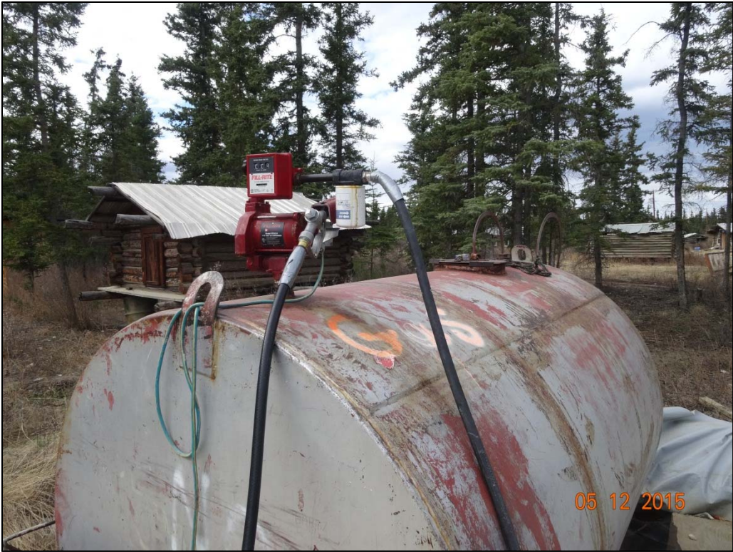
Photo 2 – Tank 1 Dispensing Pump
