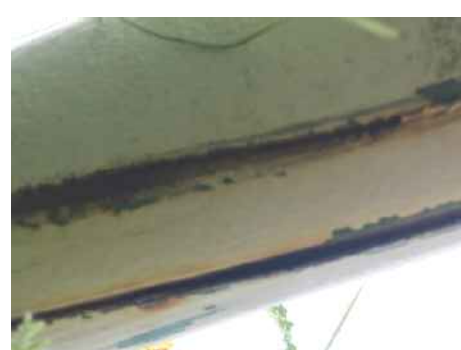
ABOVE GROUND PIPE COATING DAMAGE
