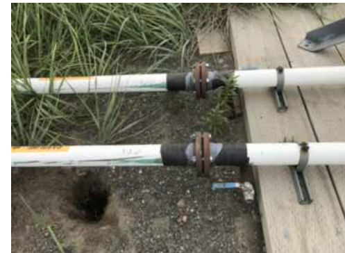
PIPE FLANGE CONNECTION AT BARGE HEADER
