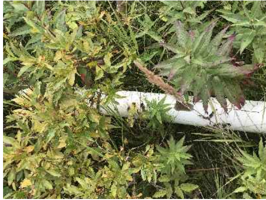
ABOVE GROUND PIPE COATING DAMAGE
