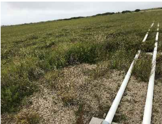
ABOVE GROUND PIPING NEAR TANK FARM
