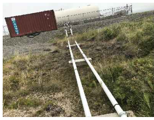
ABOVE GROUND PIPING AT TANK FARM
