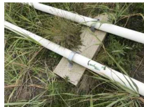
ABOVE GROUND PIPE COATING DAMAGE AND TUNDRA PIPE SUPPORT
