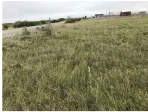
ABOVE GROUND PIPING NEAR TANK FARM - SUNKEN INTO TUNDRA
