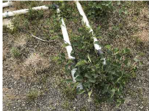
PIPING AT ROAD CROSSING
