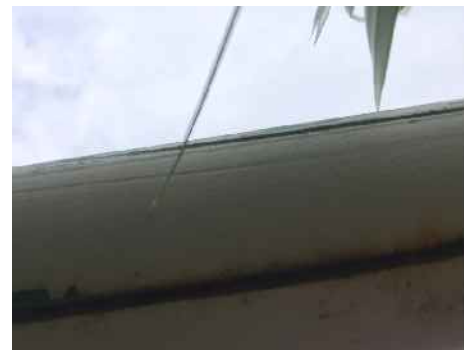
ABOVE GROUND PIPE COATING DAMAGE
