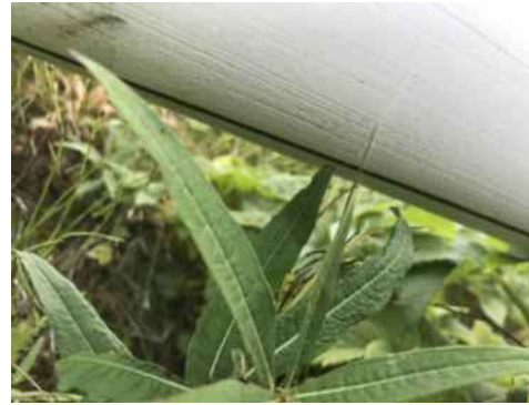
ABOVE GROUND PIPE COATING DAMAGE
