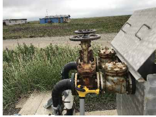
SPILL BOX AND BARGE HEADER VALVES
