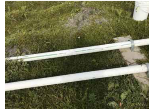
ABOVE GROUND PIPE COATING DAMAGE
