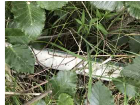
ABOVE GROUND PIPE COATING DAMAGE
