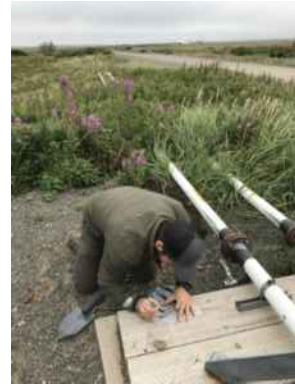
ABOVE GROUND PIPE
