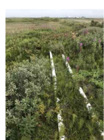
ABOVE GROUND PIPE
