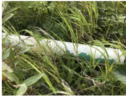
ABOVE GROUND PIPE COATING DAMAGE
