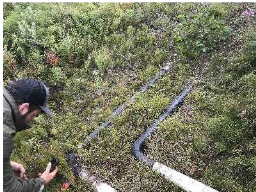
PIPING AT ROAD CROSSING
