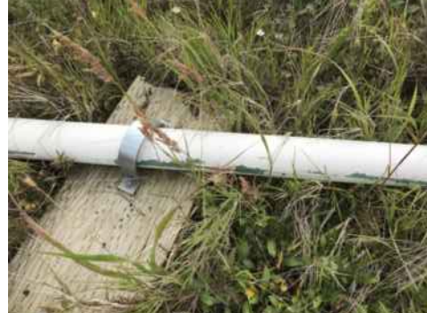
ABOVE GROUND PIPE COATING DAMAGE
