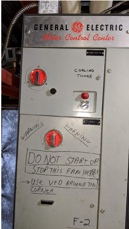
Penthouse Motor Control Center
