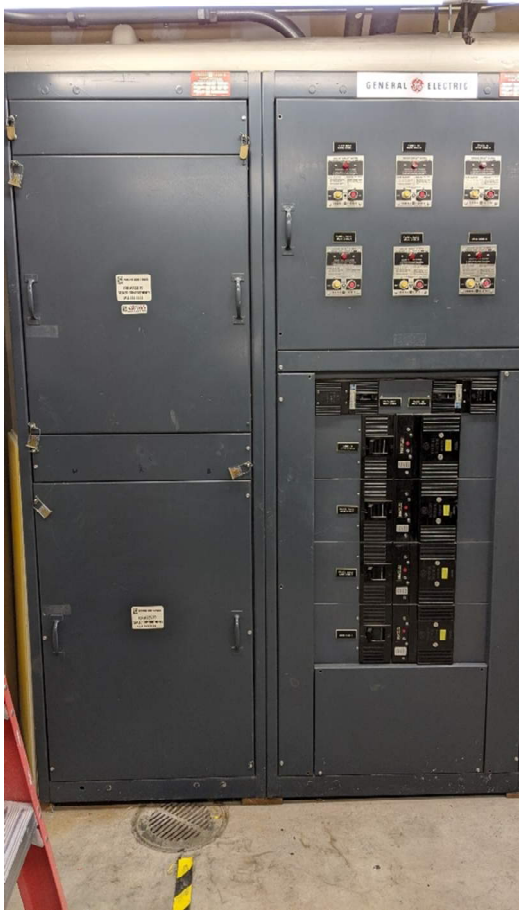
MDP in Basement Electrical Room
