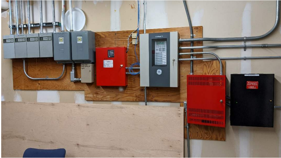
Main Fire Alarm Panel
