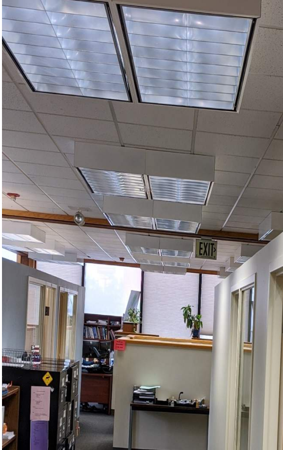
Emergency Bug-eye and exit sign.
