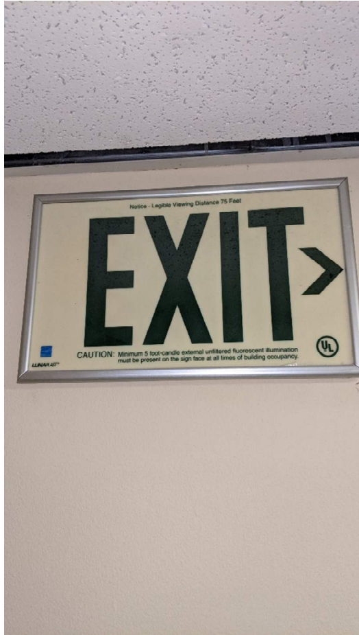
Photoluminescent Exit Sign
